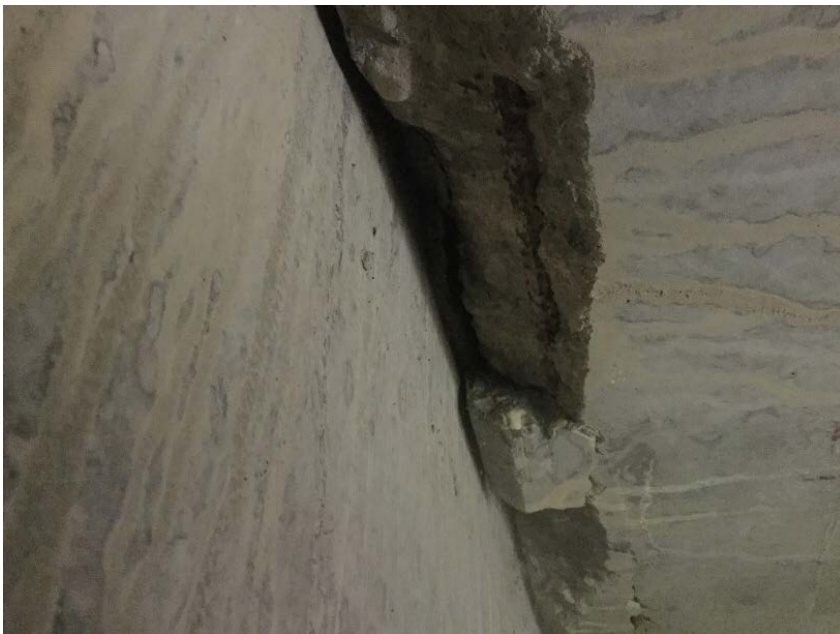
Damage to panel 1 on RB, limited to underside
