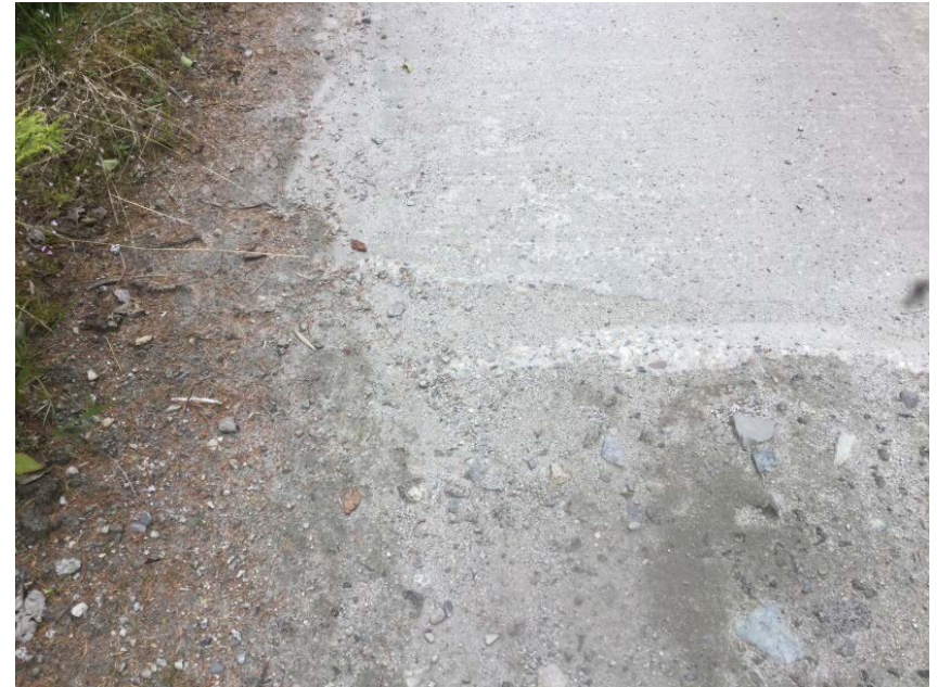
Deck and ballast wall damage on left bank
